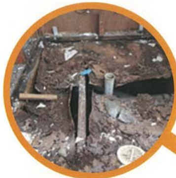
FAILED WATERPROOFING MEMBRANES IN SHOWER RECESSES
